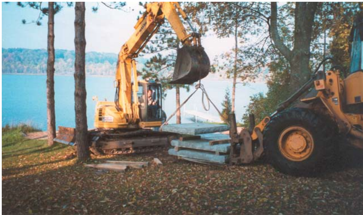
Pavers may be placed using slings. After placing paver & removing slings, one may nudge pavers into their final position with an excavator.
